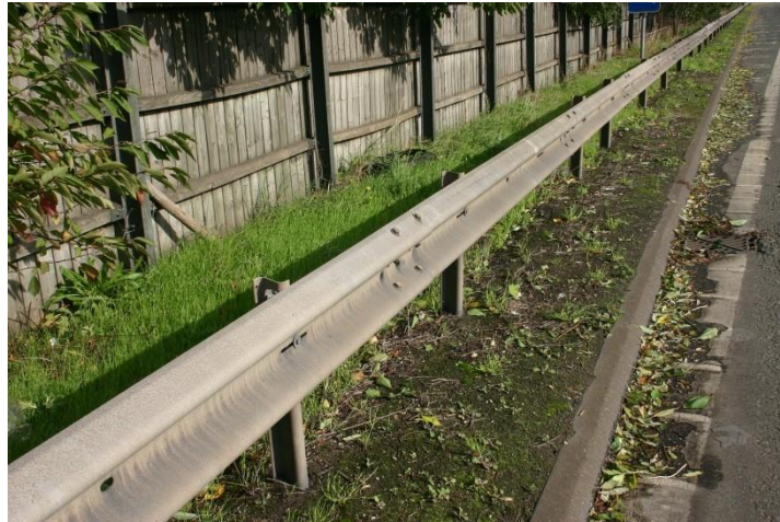
Figure 1 Steel Safety Barrier
