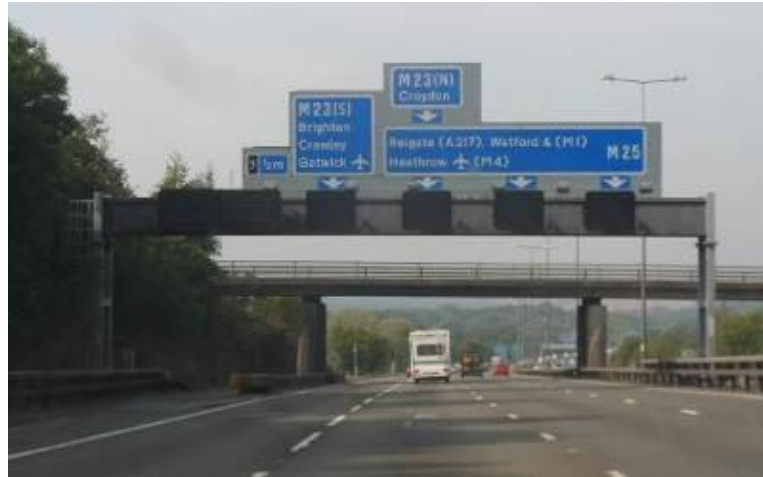
Figure 10 Typical portal gantry (two legs)
