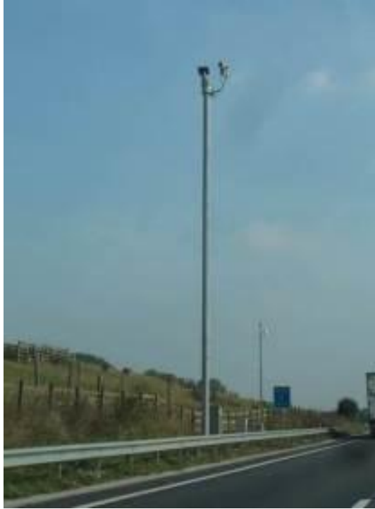
Figure 12 Typical mast mounted CCTV camera
